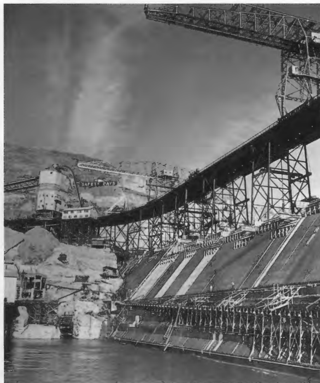
Grand Coulee Dam Under Construction on the Columbia River, 1939 Located in central Washington State, Grand Coulee was one of the most ambitious projects of the New Deal's Public Works Administration. It is the largest concrete structure in the United States, and the central facility in the Columbia Basin Project, which generates electricity for the Pacific Northwest and provides irrigation for half a million acres of Columbia Valley farm land—services that have transformed the life of the region.
